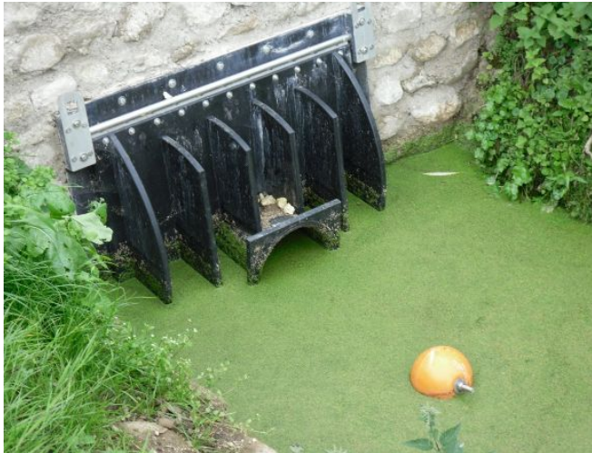
An installed flap valve showing the open 'pet flap' allowing some flow on the rising tide.
